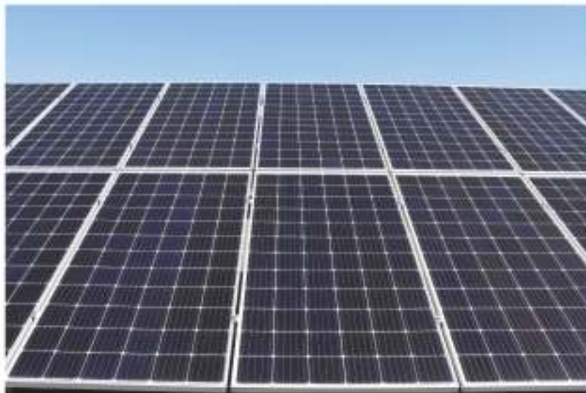
Figure 6 Photovoltaic Panels (Source: LCEC from Pixabay)
