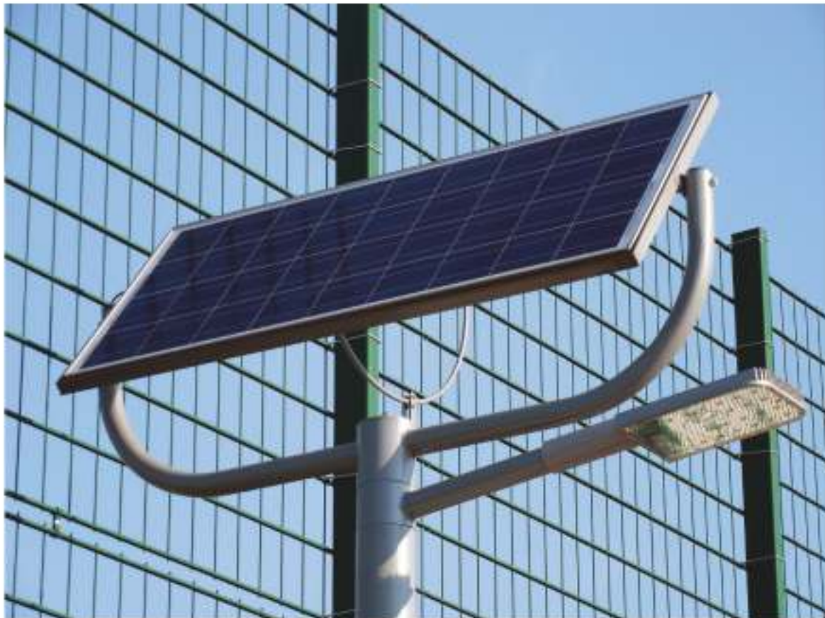
Figure 5 Solar Lighting and Fencing (Source: Succo from Pixabay)
