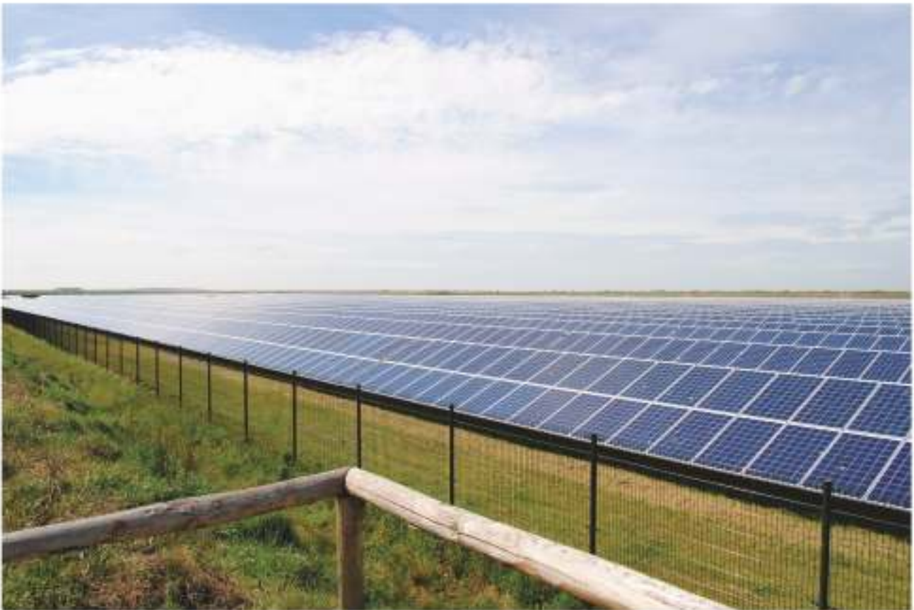
Figure 2 View of Solar Arrays (Source: AB27 from Pixabay)
